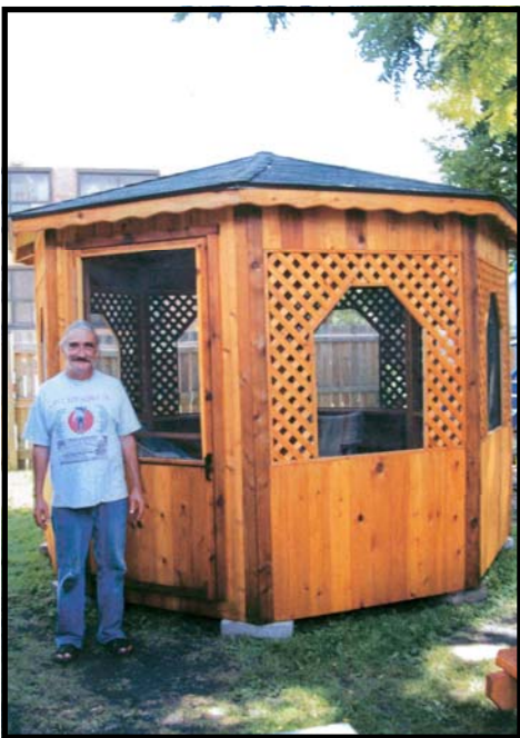
Lloyd (Maintenance) puts together a gazebo for the Haven of HOPE safe home purchased with help from the Mary Kay Foundation.
